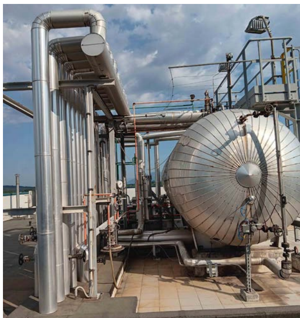
Figure 3. Expansion vessel inert gas.
