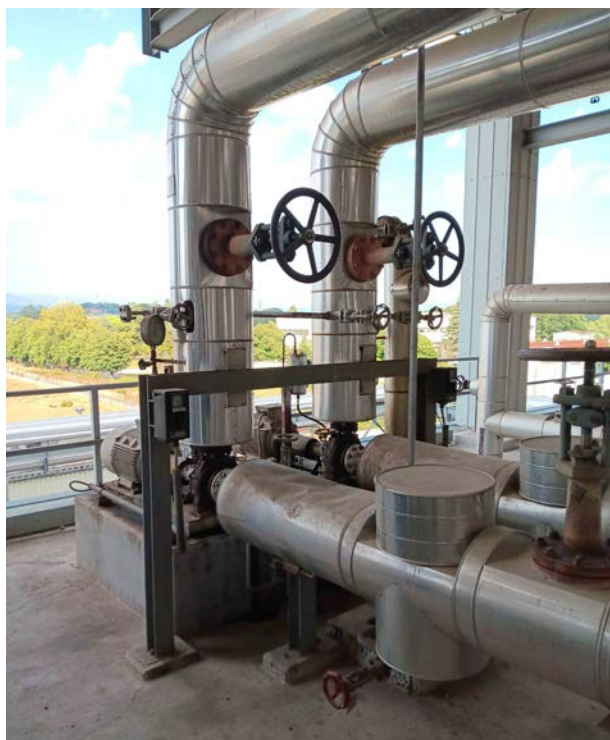
Figure 1. Secondary circuit pumps.
