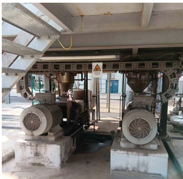
Figure 4. Primary circuit pumps.
